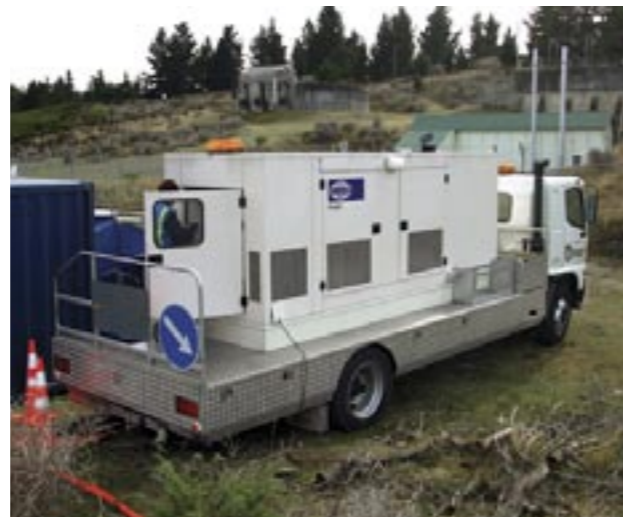
Above: In late March 2006 Orion worked with Transpower to maintain electricity supply to local residents during a major upgrade to Transpower's Coleridge grid exit point. We arranged and supplied equipment, including one of our mobile diesel generators.
