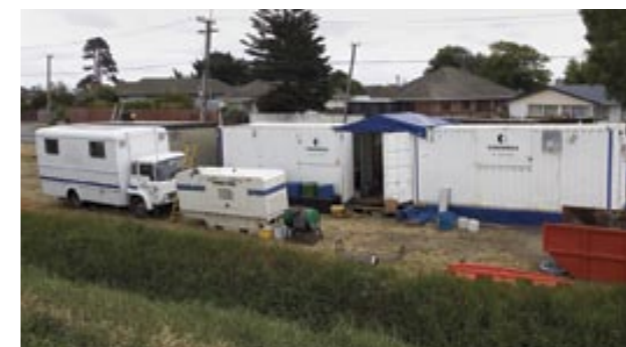
Above and right: 66kV cable joint replacement work undertaken by our subsidiary company, Connetics.
