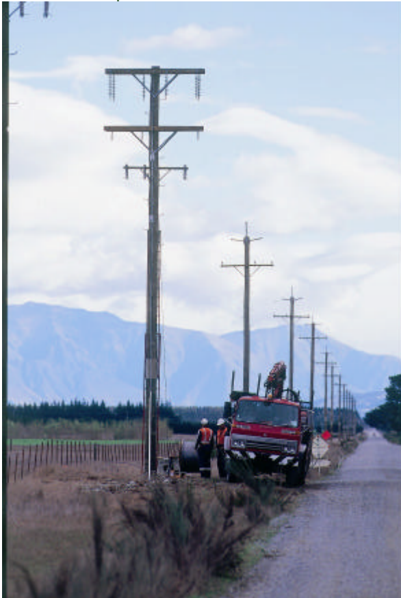
More than $8m is being invested to upgrade the rural network in the next 3 years. The growth of electricity use for irrigation is driving the investment.
