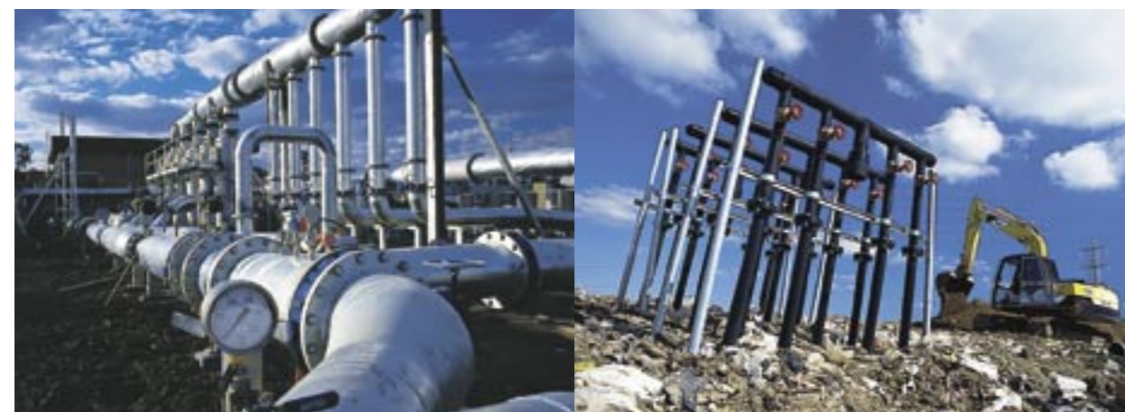
Two projects by Energy Developments Limited (left to right): Coal mine waste methane gas processing prior to use in engines at Appin Power Plant, Australia; and a well station at one of the company's landfill gas power generation facilities.
