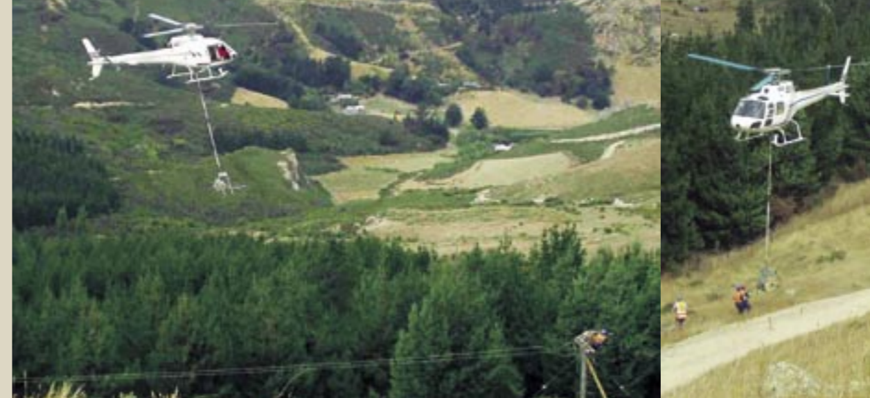
Installing lines and cable to the first wind turbine on Banks Peninsula, at Gebbies Pass.
