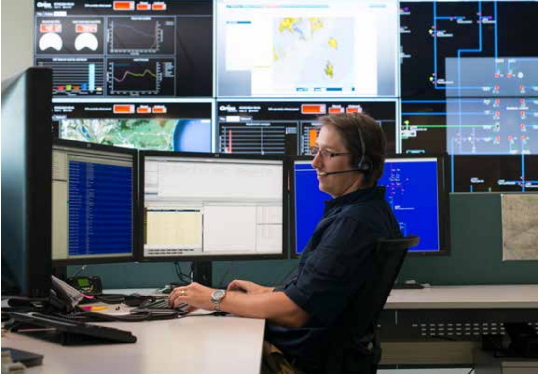
Above: Our 24 hour control centre is the hub of our network operations. Ian Ainsworth, Network Controller, is part of the team who monitor and control our network.
