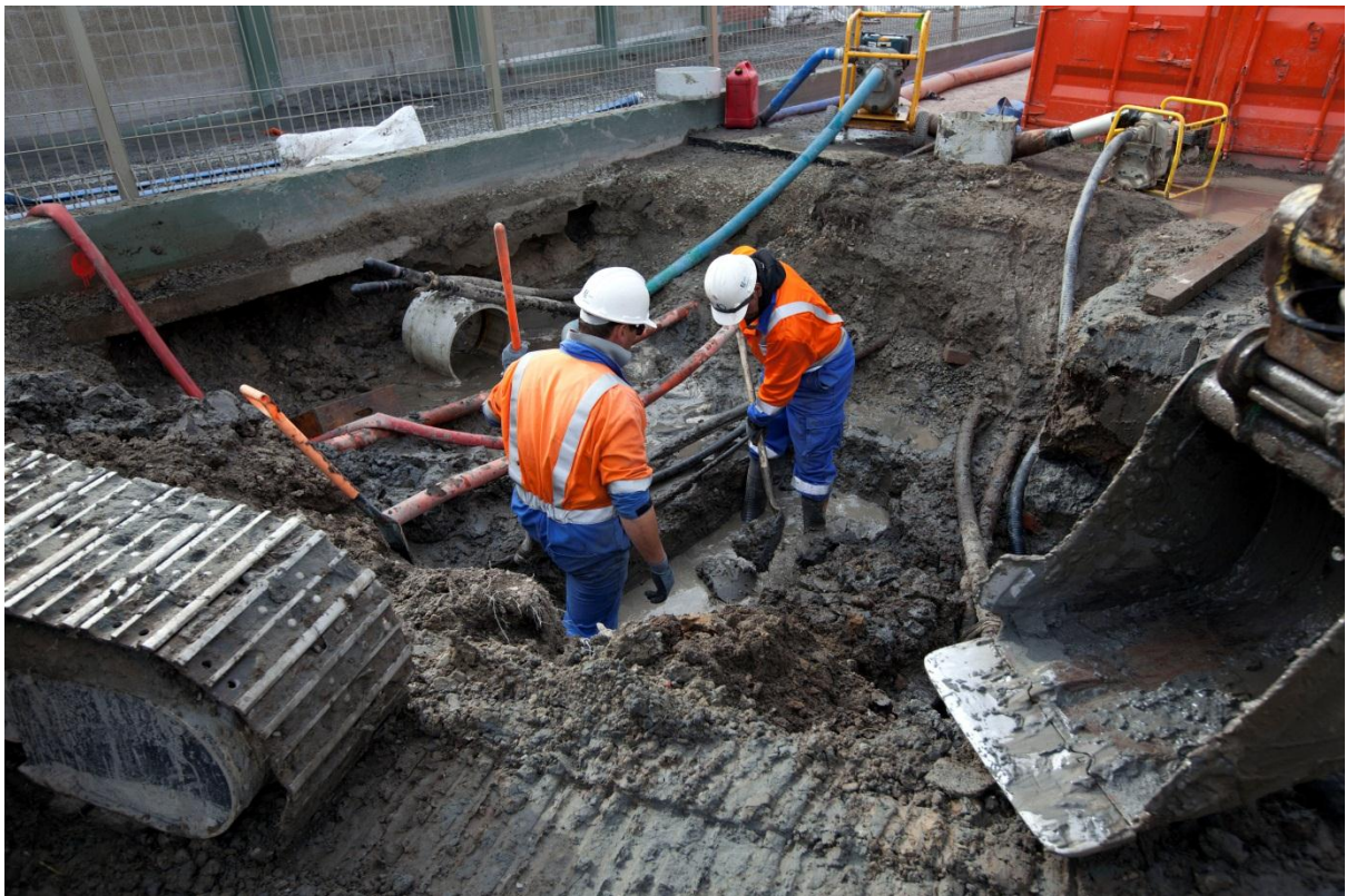
Orion contractors replace damaged 11,000 volt cables in New Brighton following the February 2011 earthquake.
