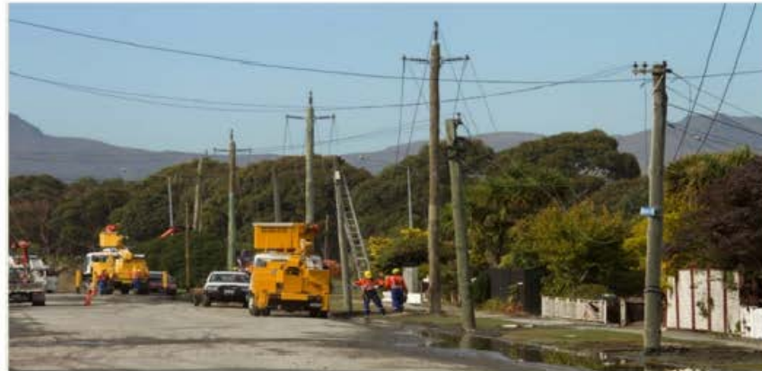
Figure 29: Emergency 66kV Overhead Line
