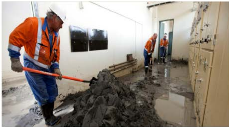
Figure 18: Liquefaction Inside Major Substation
