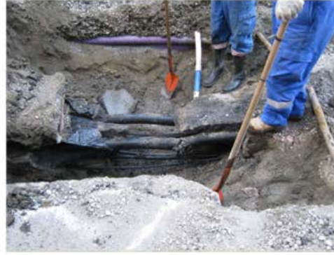
Figure 14: 66kV Oil Filled Cable Damage – Armagh Street
