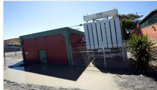
Figure 17: Liquefaction Impact on Major Substation
