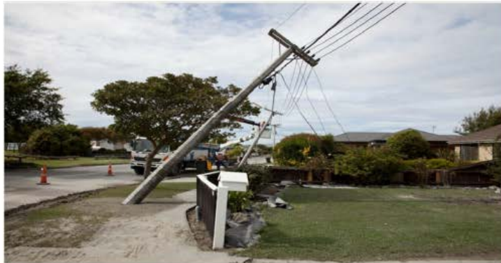
Figure 16: Low Voltage Line Damage
