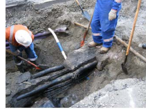
Figure 15: 66kV Cable Damage
