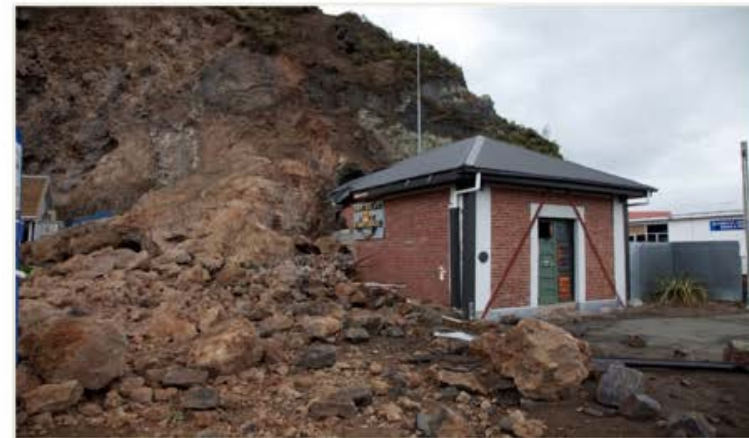
Figure 21: Substation Rock Fall Damage
